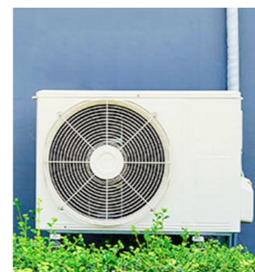
Figure CP.48. Ground & Air Source Heat Pumps
