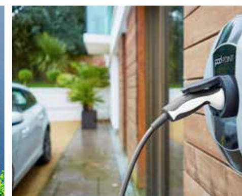
Figure CP.49. EV charging point at home
