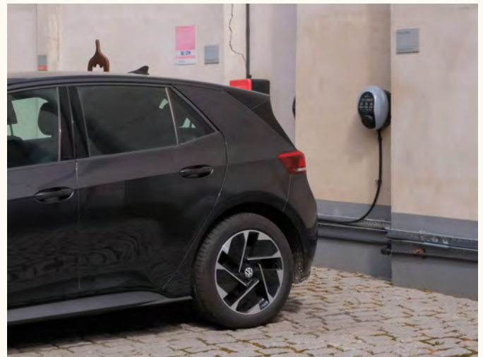
EV charger integrated into street furniture and a discreet wall-mounted charger.
