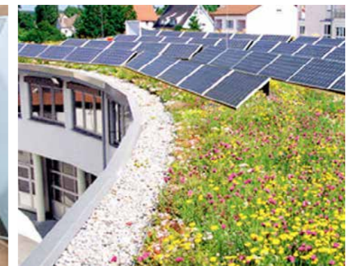
Figure CP.50. Solar Photovoltaic Panels
