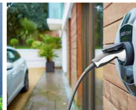
Figure CC.81. EV charging point at home
