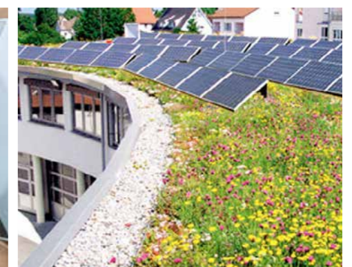
Figure RA.29. Solar Photovoltaic Panels
