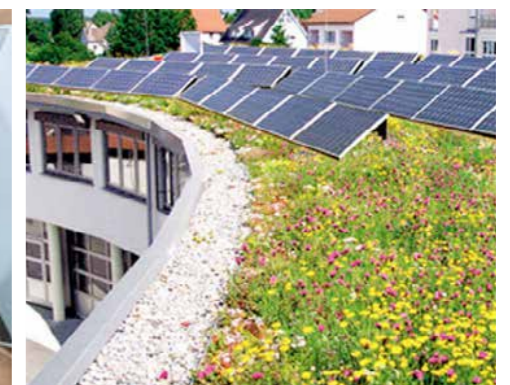
Figure CC.82. Solar Photovoltaic Panels
