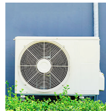
Figure CC.80. Ground & Air Source Heat Pumps
