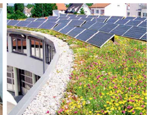
Figure VA.70. Solar Photovoltaic Panels
