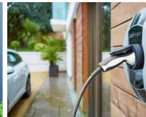
Figure CP.49. EV charging point at home
