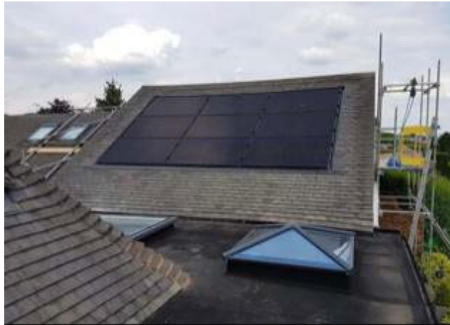
Solar panels sitting flush to the roofline on a property in Shenstone
