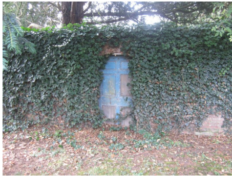
Picture 8.1 Lack of maintenance increases the likelihood of buildings and structures becoming at risk
