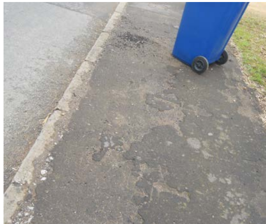
Picture 7.7 20th Century concrete slabs replacing the traditional stones along Main Road.
