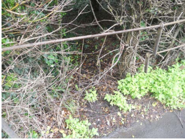
Picture 8.6 Damaged railings surrounding Haunton Hall.
