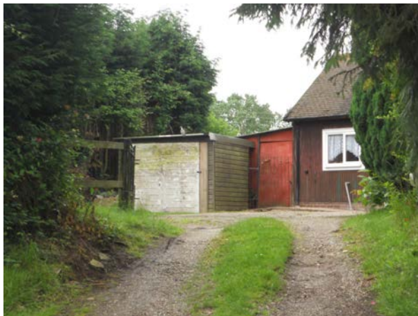
Picture 8.8 Deteriorating garage.
