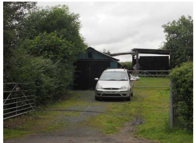
Picture 8.9 Deteriorating garage and barn.
