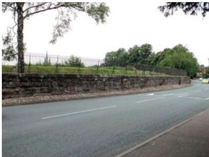
Picture 15.5 Sandstone boundary and railings to Stowe Pool showing raised level of Pool
