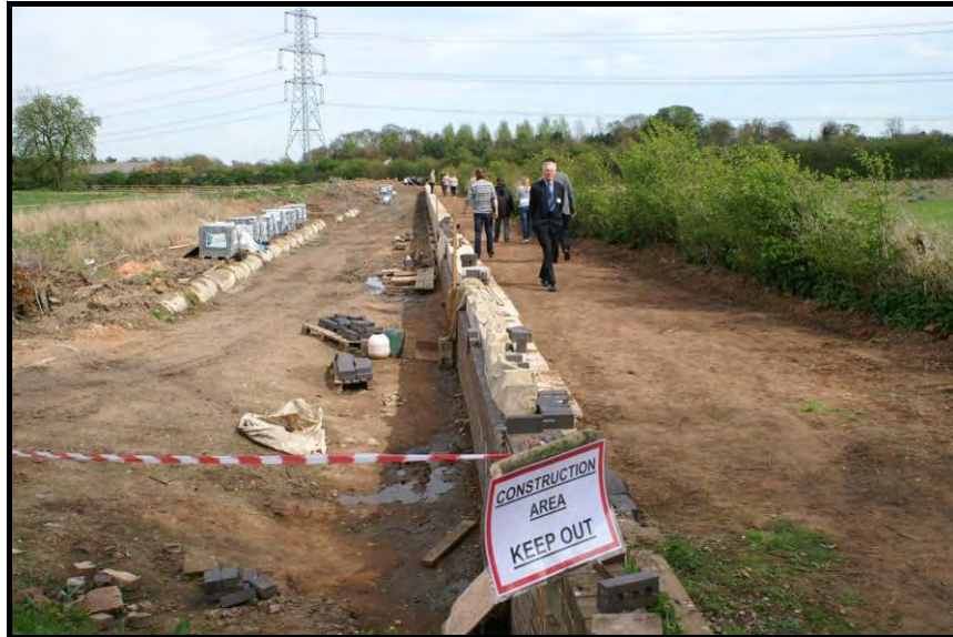
Waterway wall on south side of pond below Lock 26 under construction, seen here on the day of the opening of the Borrowcop Locks Canal Park 26
