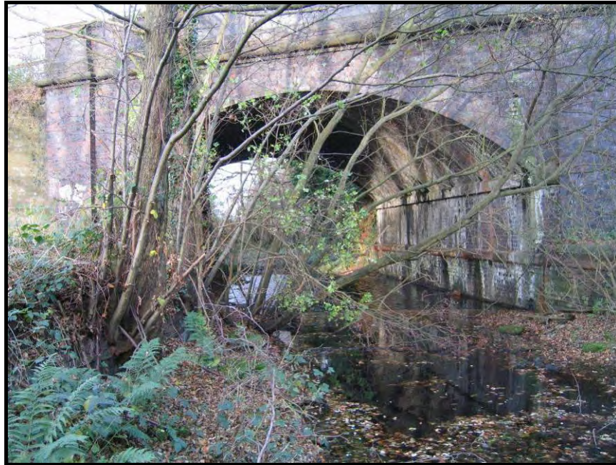
Pipehill Bridge, with shallow standing water in the bed of the canal. The photo was taken standing just under the brick towpath side waterway wall, which is generally quite well preserved on this side of and under the bridge.
