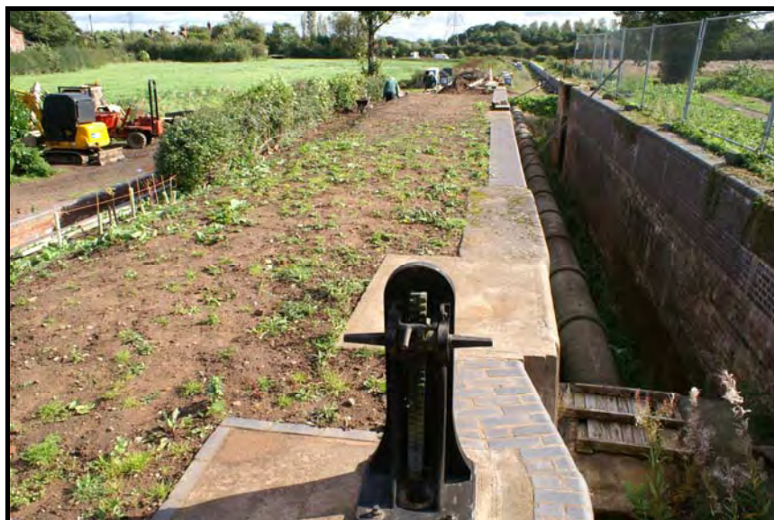
Lock 26, under restoration by the Trust. The piped land drain can be seen in the bottom of the lock chamber 27
