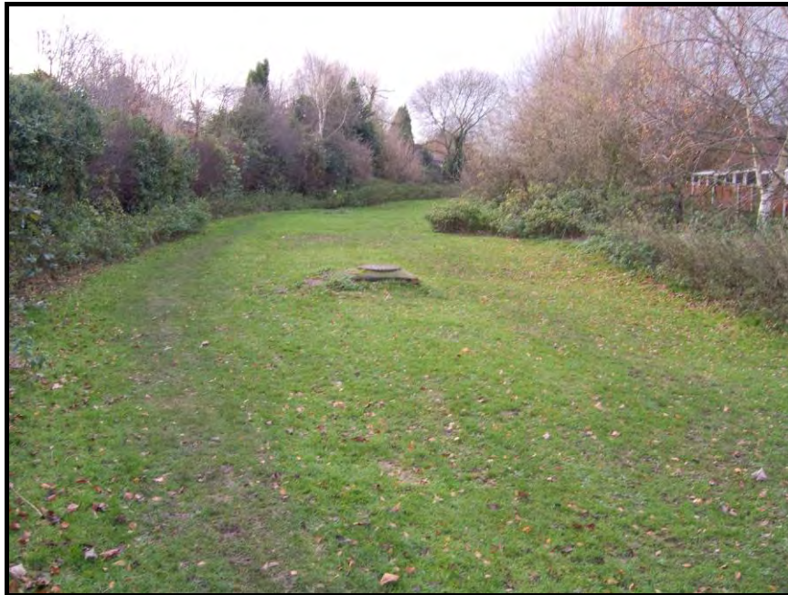
Section of alignment between proposed footbridge site and London Road. Culverted land drain chamber is visible in centreframe.
