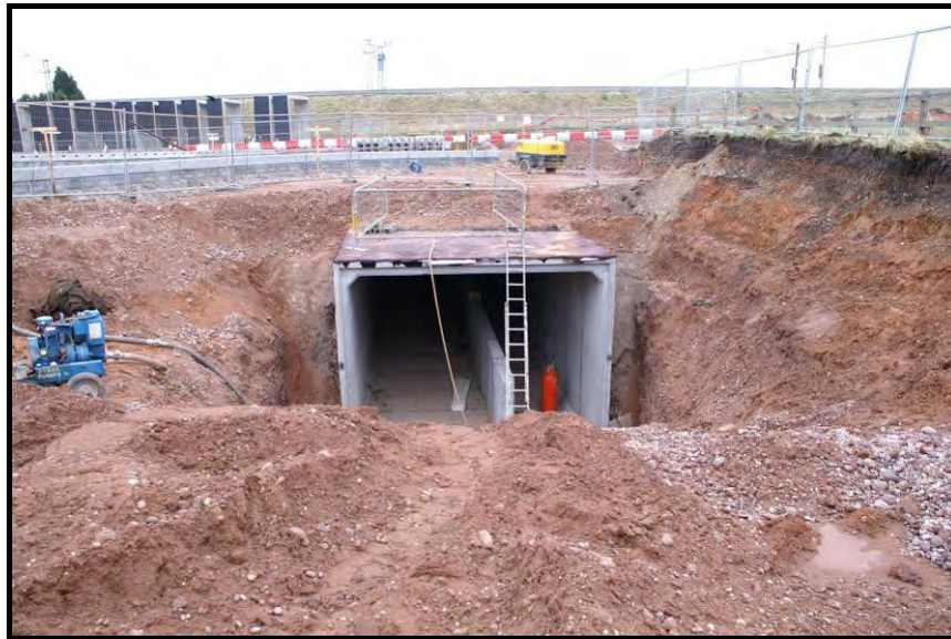
The Birmingham Road Culvert under construction (now temporarily buried). This is taken from a very similar viewpoint to the photo above. 30
