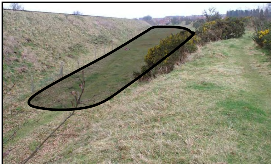
Trust land west of the railway turn – the gorse covered bank to the right (south) of the Trust land is the original offside bank of the canal. 33
