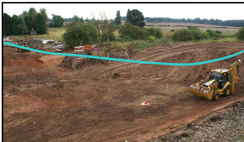
The railway turn, seen from the freight railway embankment. Site clearance work is underway for the Southern Bypass, and the bottom end of the former Lock 19 has already been demolished. The proposed route for the canal is marked. 32
